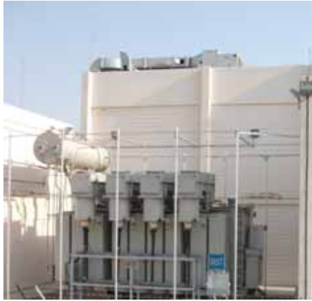
• 67MVA, 110kV Al-Haramain
