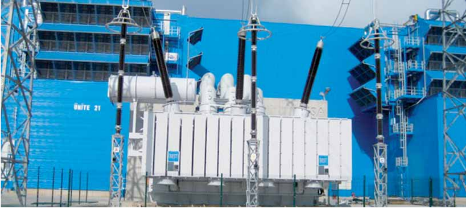
• 310MVA, 400kV GSU Transformer in Antalya CCPP
