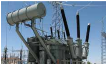
• 250MVA, 380kV Autotransformer - TEİAŞ
