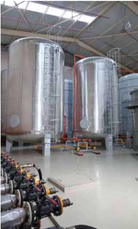
• Oil treatment plant
