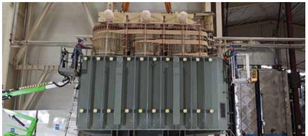
• The active part being placed into the tank
