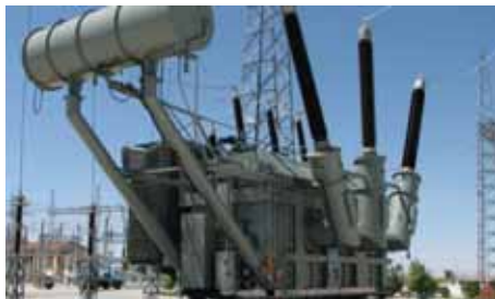
• 250MVA, 380kV Autotransformer - TEİAŞ
