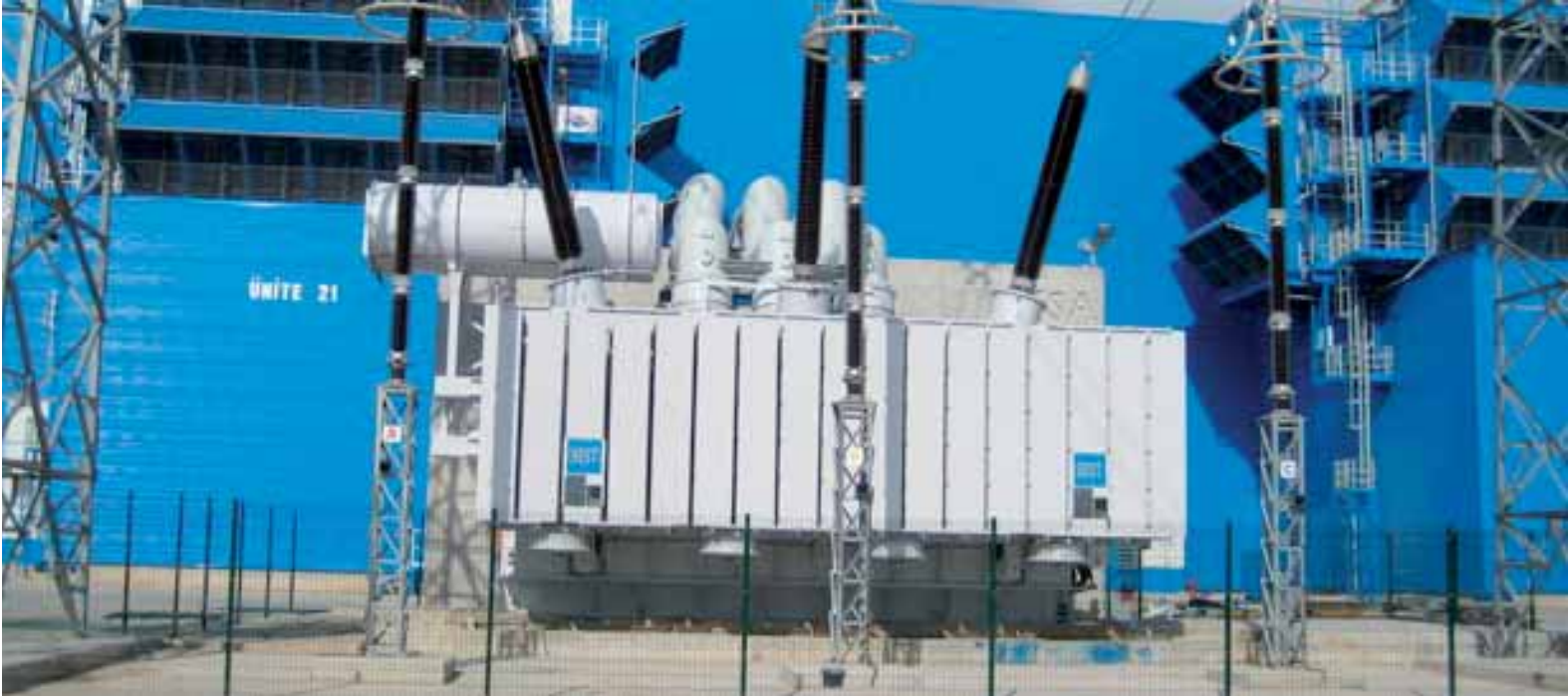
• 310MVA, 400kV GSU Transformer in Antalya CAPP
